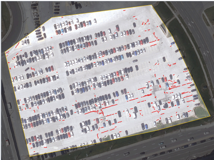
Crack-like lines traced on the 2023 imagery (red); paved outline in yellow; areas outside it dimmed.
